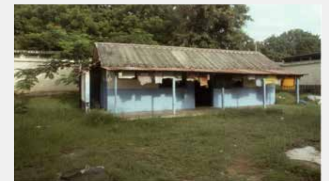
Figure 4a: How to build a paediatric ITU in three months in Kilifi Kenya, 1990 (before)
